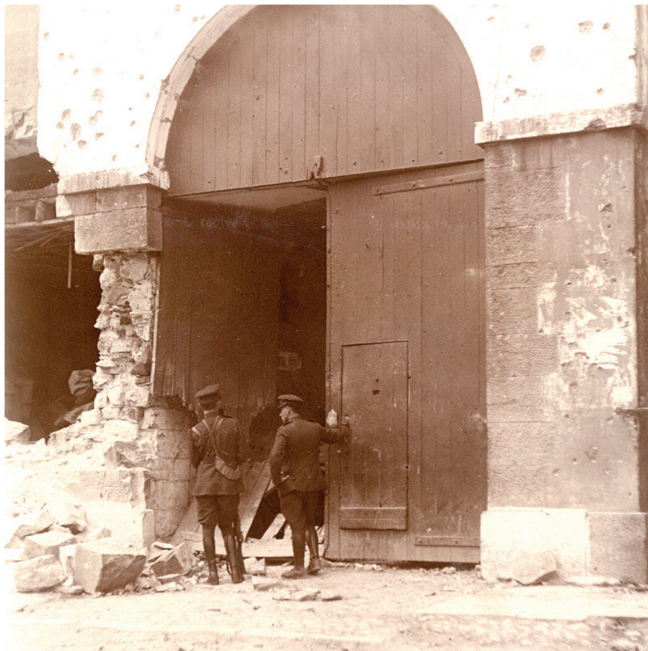
Fig. 49, Soldiers examining the damage to Strand Barracks, c. 21 July 1922
